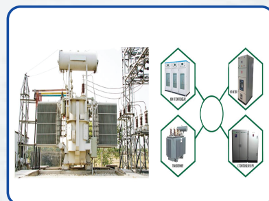
Transformer/DB/SDB Switchgear/ Substation
